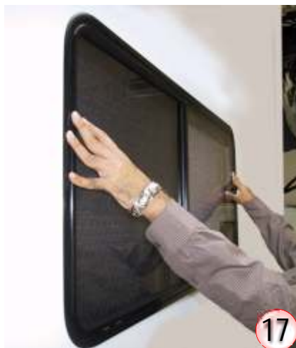
One person needs to hold window from the outside of the van.
