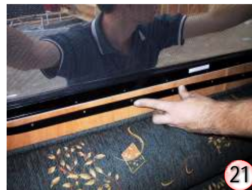
Position clamping around the window in the same as when holes were drilled.
