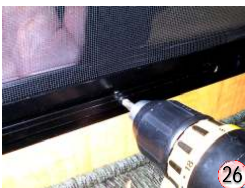
Fasten 2 bottom screws. Window is now secured. The outside can now be allowed to sit in place. The rest of the screws can be installed from the inside. Remove excess silicone or any other be sealing compound - general cleanup.
