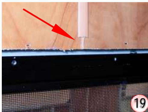
Top of window. T-section cut out the same height as the clamping.
