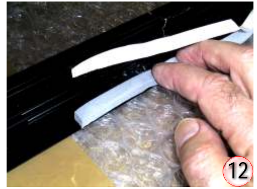
Clean dust and dirt from around the opening where the window is going to be fitted. Wipe window main frame flange with a dry cloth to remove dust. Apply sealing compound to flange. Foam tape is used in this case in the above picture.
