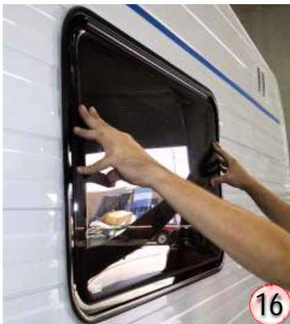
One person needs to hold window from the outside of the van until a second person starts reinstalling the clampring to the window from the inside of the van. Clampring must be reinstalled in exact position for the holes to match up.
