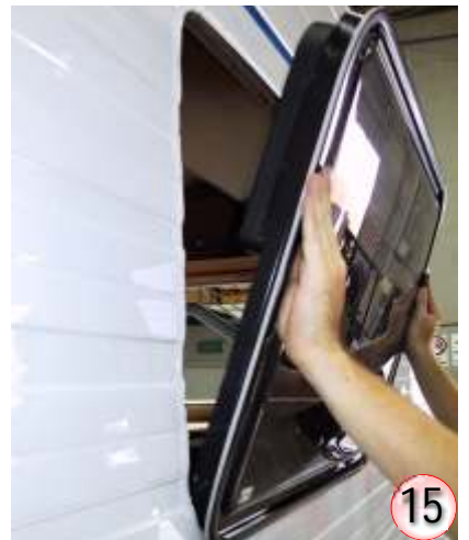
With the bottom of the window in place, gently push the top of the window in position in the opening.
