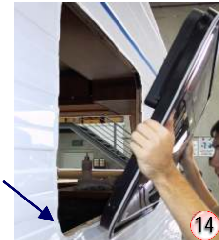
Fill seams with silicone then crush. Position window in opening on the wall of the van where it is going to be permanently installed. Do this from the outside of the van. Note! Bottom of the window to go in first - to clear thumb locks.
